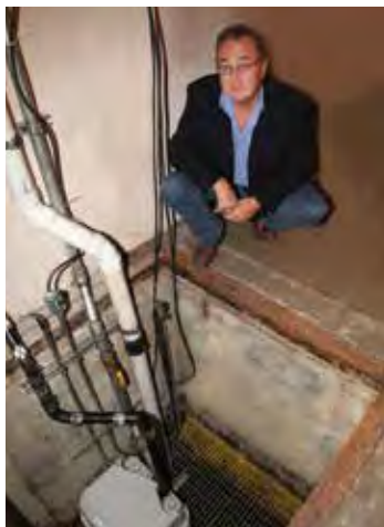
Sanicubic 2 grinder pump installed inside a pit where several bathrooms drained into the pump
