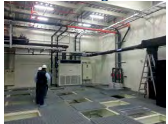
Mechanical room with two Sanicubic 2 grinder pumps installed
