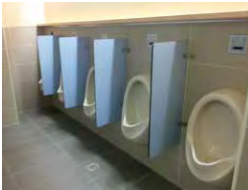
Several fixtures are discharged into Sanicubic 2 systems
