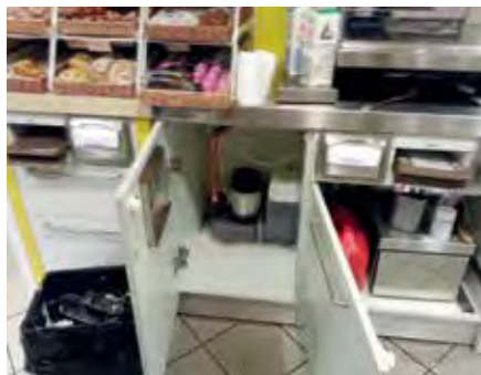
Sanicom installed inside a cabinet with easy access
