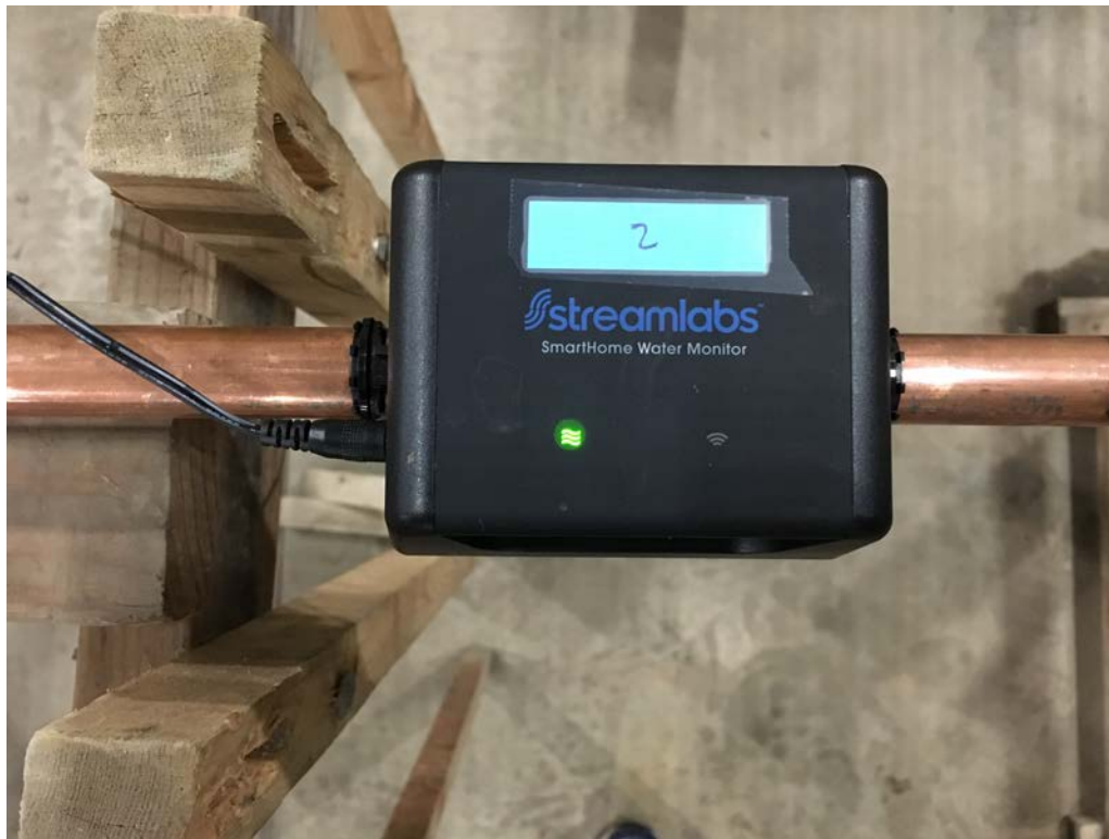
Streamlabs Water Monitor on copper pipe
