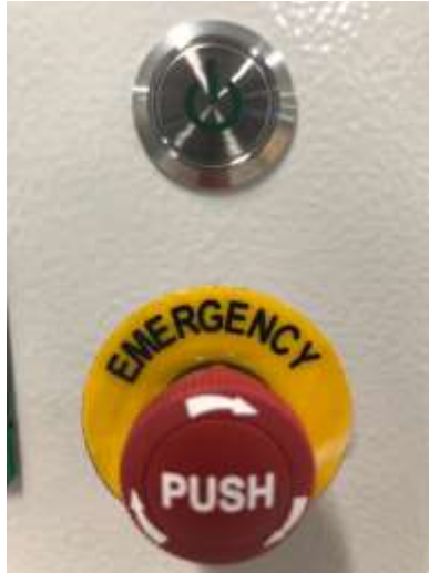
Figure 5: The Power button and estop are not activated
