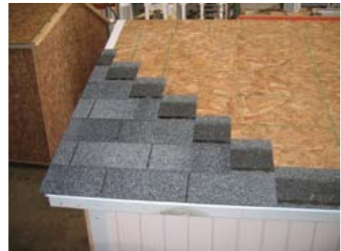
Cut ridge cap in the shape shown in picture and start to place the cap on the top of the building.
