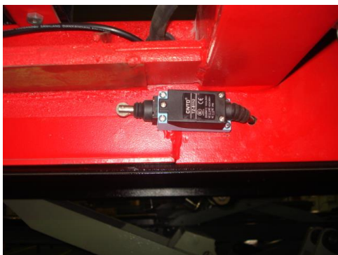
Picture 23 (main lift up limit switch)
