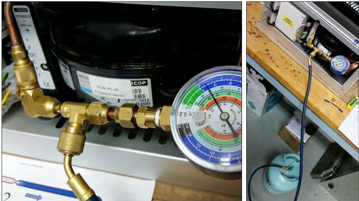
Figure 4-38 Hose attached to the pressure gauge and to the cylinder of R134a
