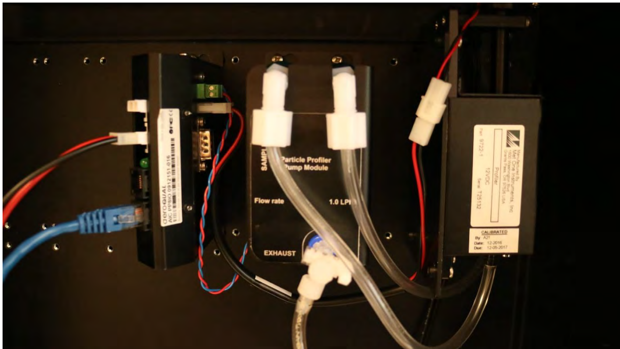
Figure 1-17 An update to the pump module with the filters installed inside the pump module
