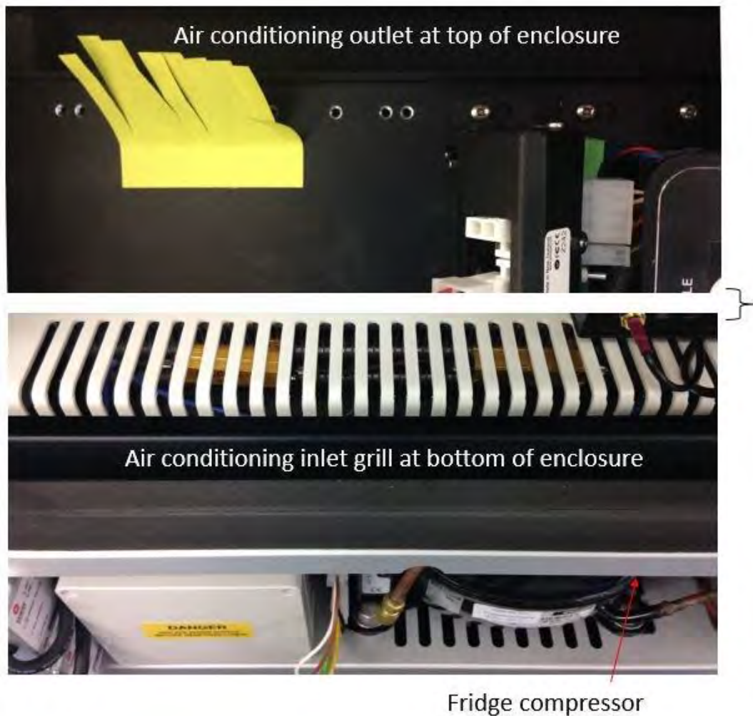
Figure 1-20 Air conditioned air is constantly circulated in the AQM 65 enclosure. Air comes in to the enclosure at the top and exits through vents at the bottom
