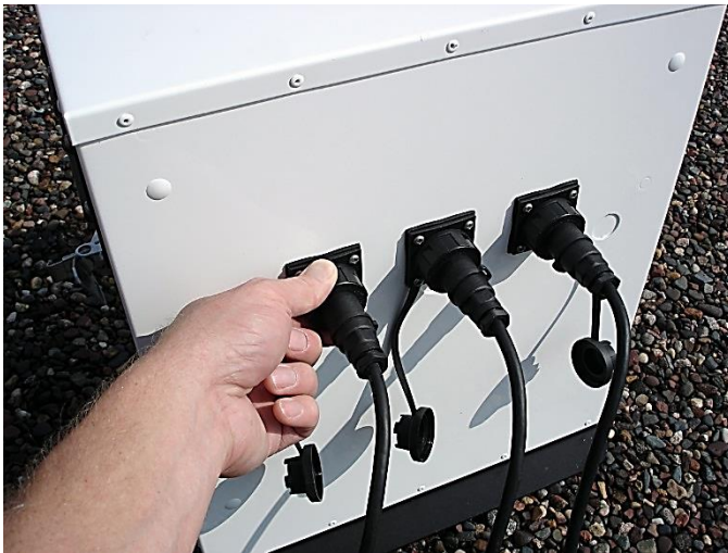
Figure 39: Connect Power from the Solar Cell Power System to the Environmental Enclosure
