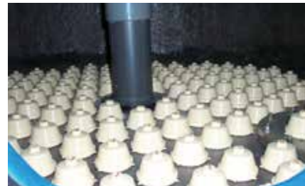
Nozzle Plate under drain system
