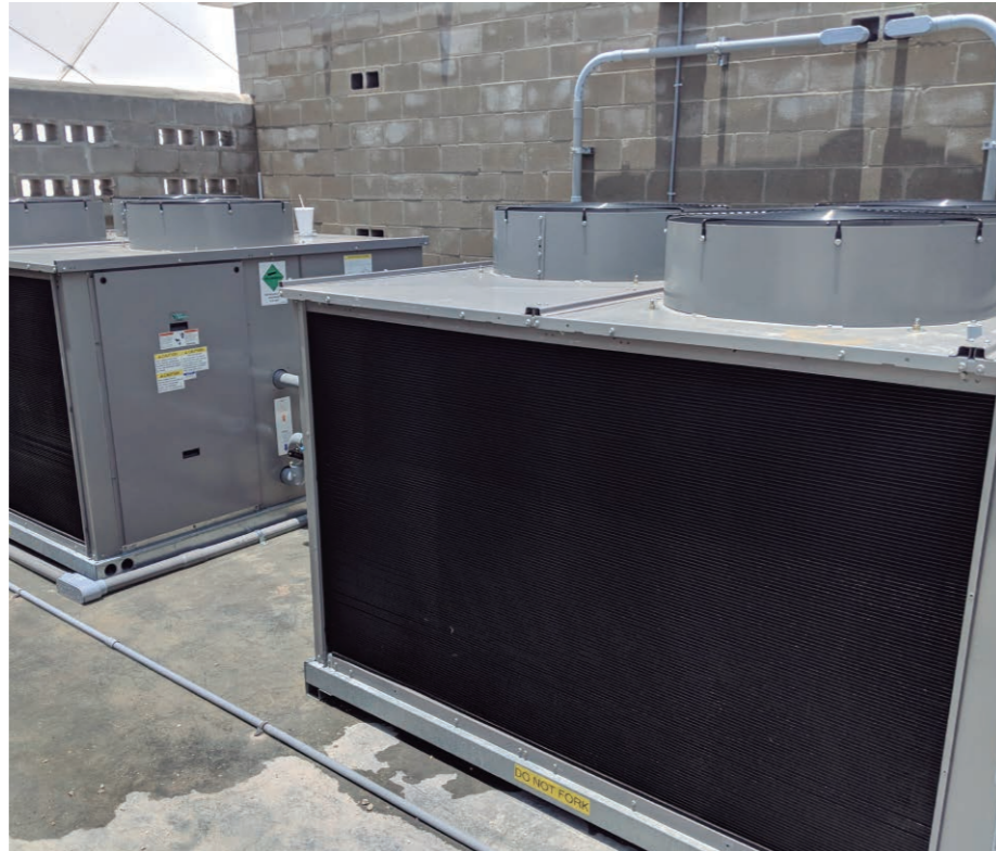
Dual Ton chillers in Shrimp farm.
