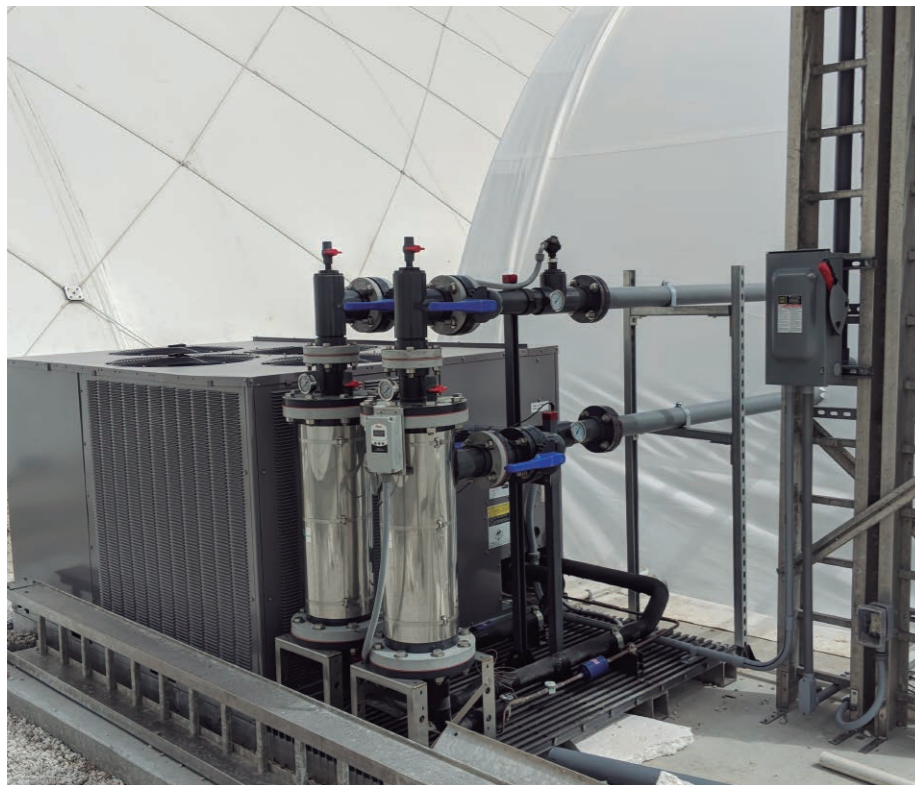
Ton chiller in shrimp farm.
