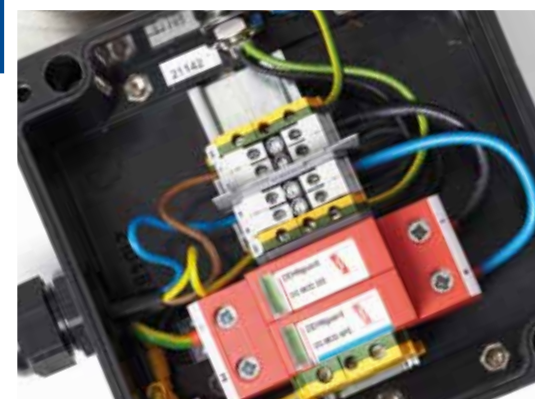
GRP junction box
