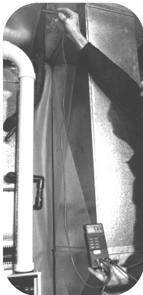
FIGURE 48 TEMPERATURE RISE MEASUREMENT
