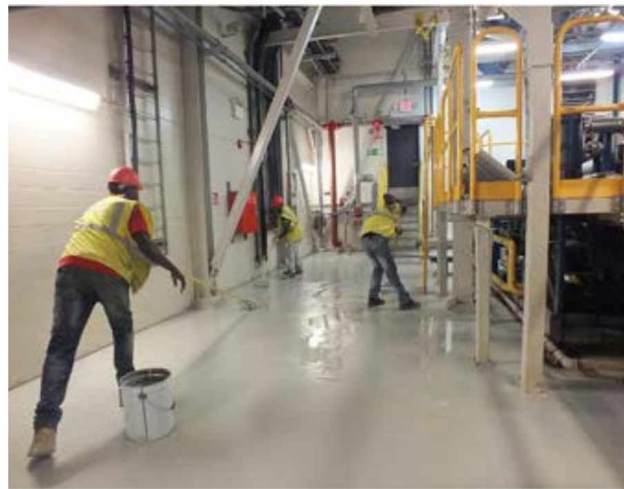
Installation of high performance floor system at Staatsolie – Suriname's National Energy, Oil & Gas Company.
