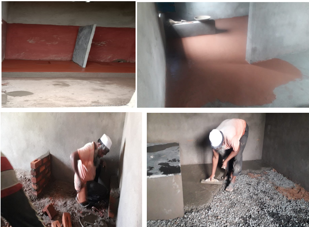
Figure 3: Repair and Rebuilding work initiated at Govt Kannada Higher Primary School, Bagalnar @ Karnataka
