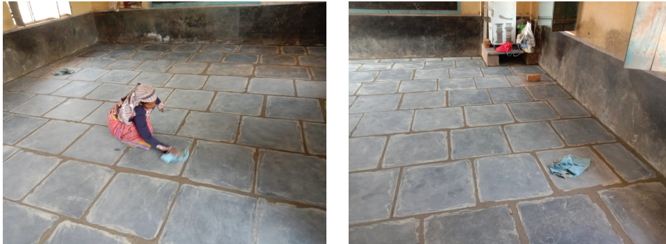
Figure 3: New flooring work getting done in one of the selected schools - Belgaum, Karnataka
