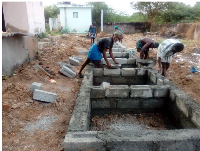
Figure 1: Bio-toilet installation at GHSS Gopalpatti, Tamilnadu
