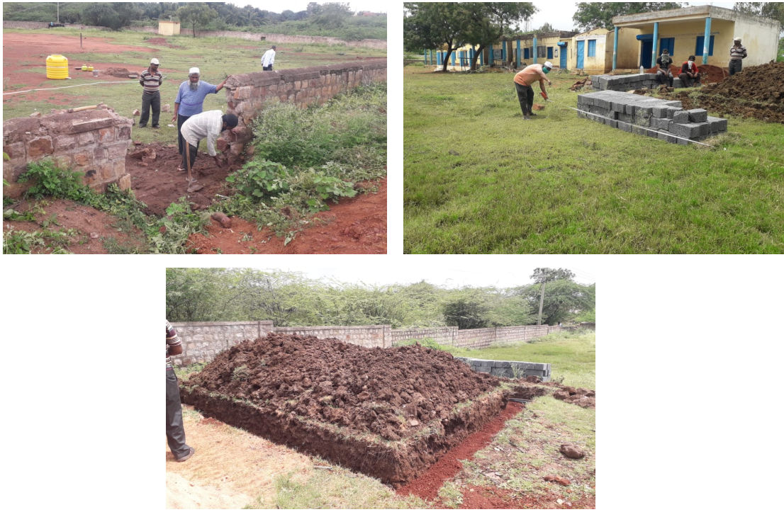
Figure 2: Repair and Rebuilding work initiated at Govt Kannada Higher Primary School, Bagalnar @ Karnataka
