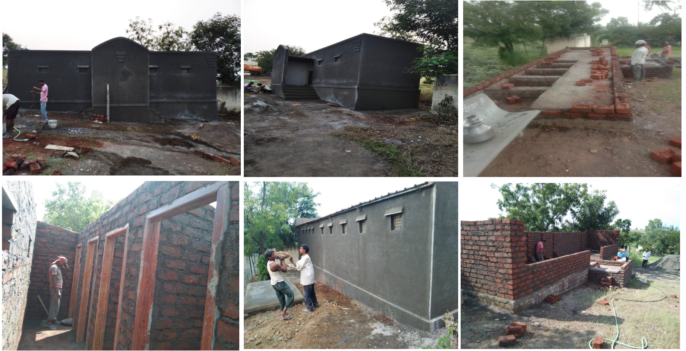
Figure 1: Sewa toilet units @ Pune ,Maharashtra
