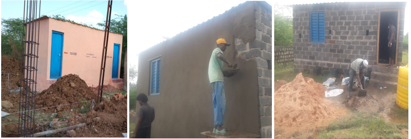
Figure 3: Repair and Rebuilding work initiated at Govt Kannada Higher Primary School, Bagarnal @ Karnataka
