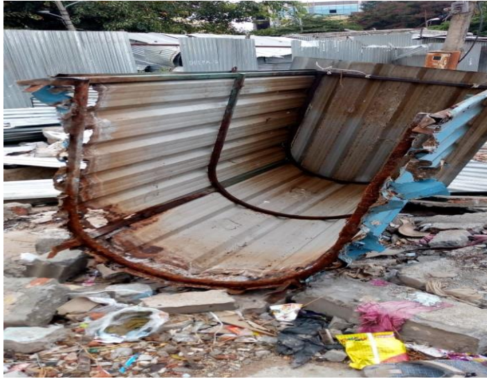
Figure 5: Rusted portable toilets after their removal at Sanjaygandhi Nagar
