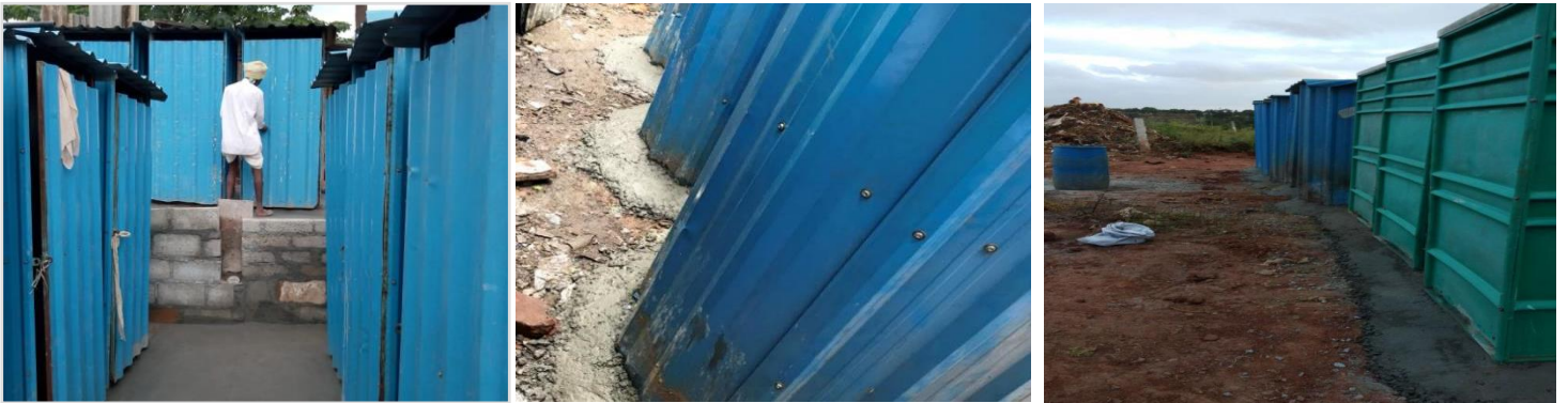
Figure 1: Reinstalled toilet units in slums of Jyothiba Phule (left), Shanti nagar (center) and JK Basavanna Nagar (right)
