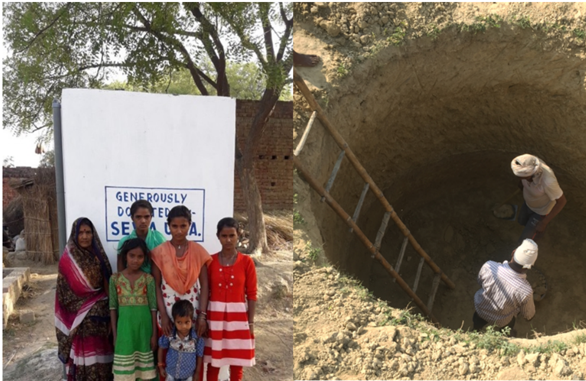
Figure 3: (left) Installed toilet @ Baluva. (Right) Villagers helping to dig the soak pits.
