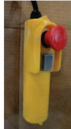
Figure 5: Red Emergency Stop Button (on Remote Switch)
