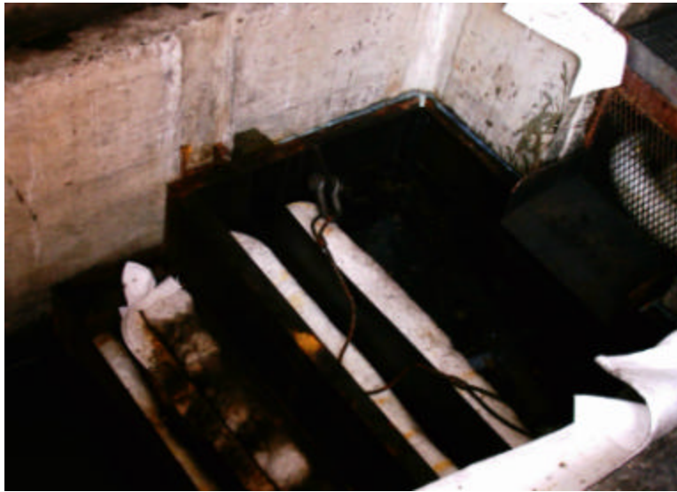
Figure 2: Oily water sump showing absorbent material and diapers for removal of the oil from water.
