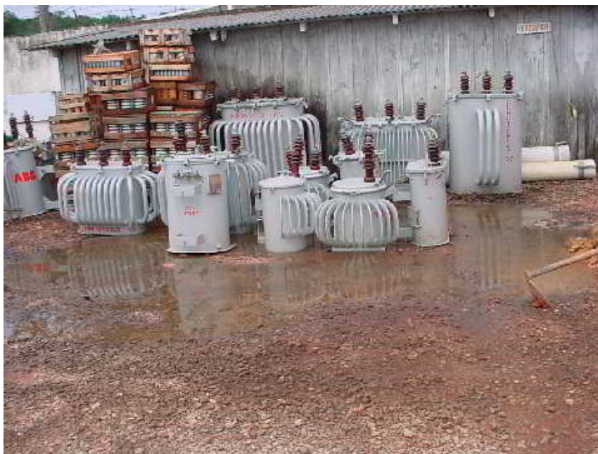
Figure 9. A substation in Mandarituba with transformers and spills
