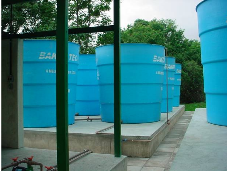
Figure 6. An array of treatment tanks
