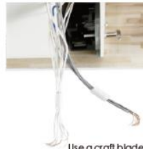
Use a craft blade to carefully skim over the plastic to bare the copper wire. Twist the same color wire together.
