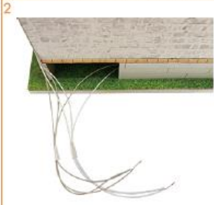
cut all the LED light wires to the same length, peel off the film of the LED light wires and then wrap it together in the same color.
