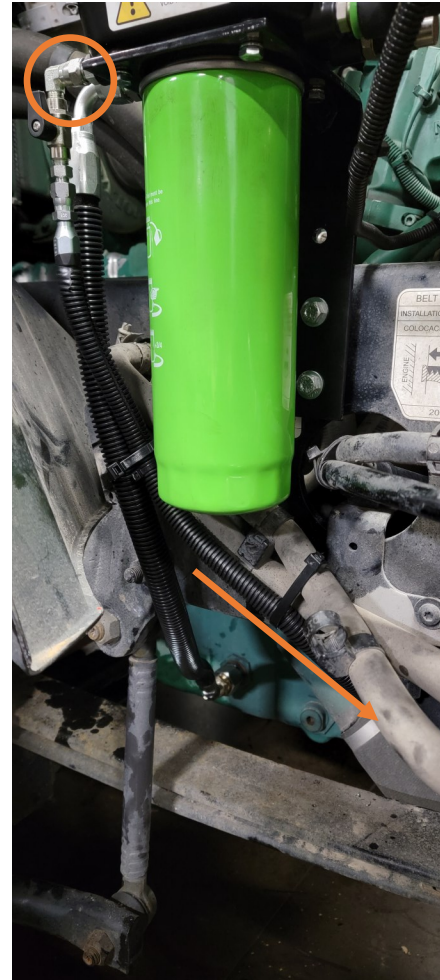
OIL FEED LINE IS RAN UNDER THE ENGINE AND ZIP TIED TO EXISTING LINES
