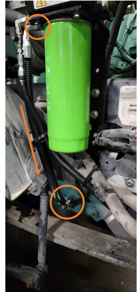
OIL DRAIN LINE IS INSTALLED DIRECTLY INTO THE OIL PAN AND ZIPTIED TO THE OIL FEED LINE FOR STABILITY.
