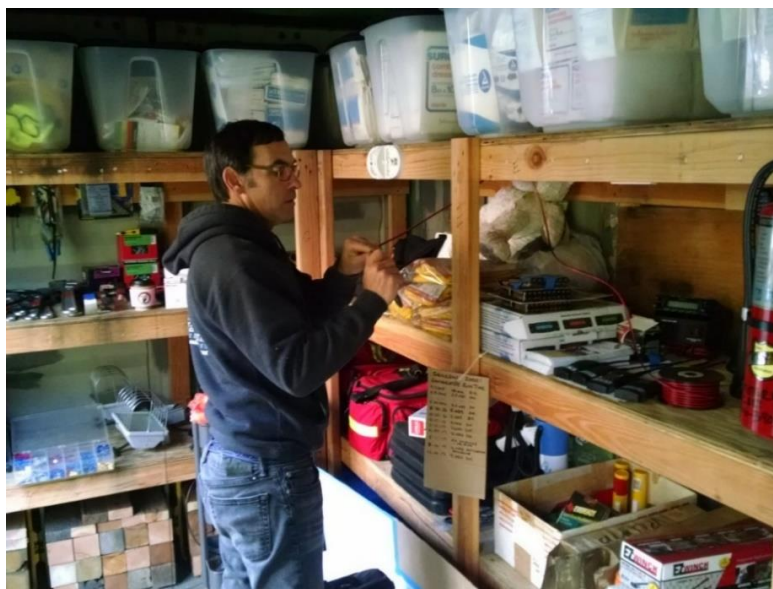
CERT Zone Captain Gene Rizzo Installs LED Lights In The Skyline Container
