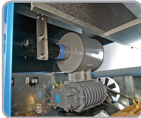
View with rear panels removed
