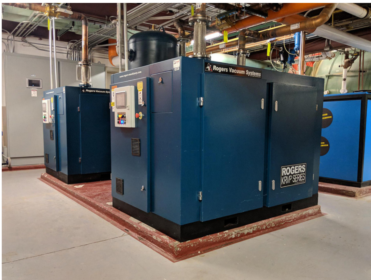
A Rogers Machinery KRVP vacuum pump installed in a facility.
