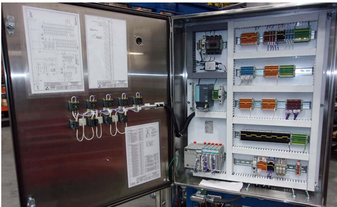
Figure 3: Low voltage control panel made by Rogers Machinery compatible with 60Hz/120VAC and 50Hz/230VAC power.
