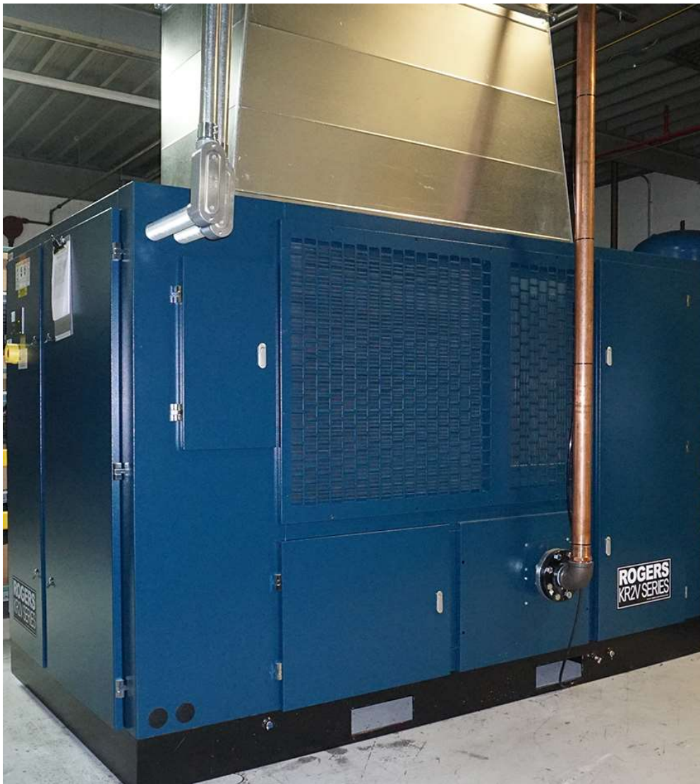
Figure 5: Installed 2-stage enclosed compressor with vertical ductwork
