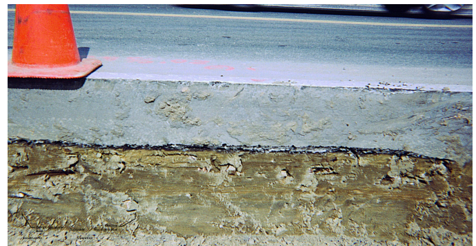
Figure 2 - Total loss of aggregate base due to contamination
