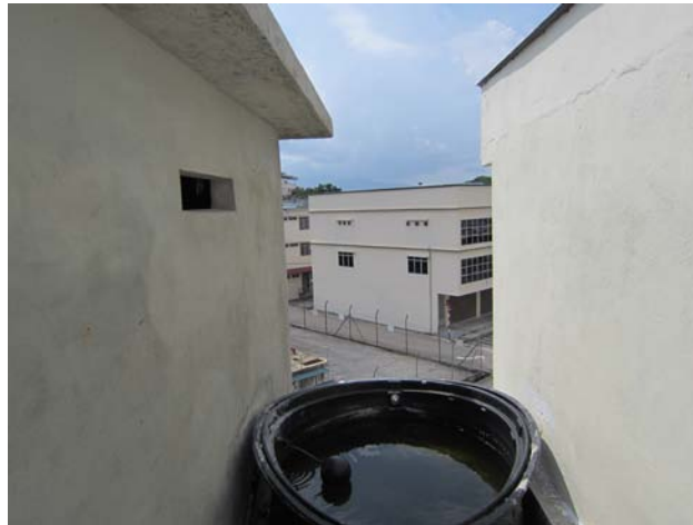
This is not an ideal entrance hole. The flight path is blocked by the monkey house next door, making swiftlet's navigation difficult.
