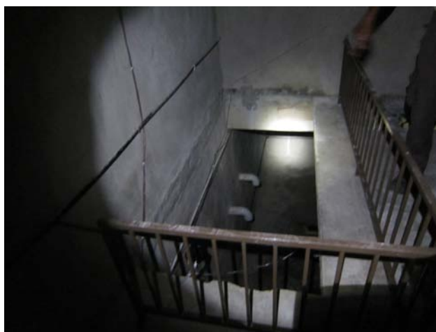
Excessively high railings obstruct the flight paths of swiftlets
