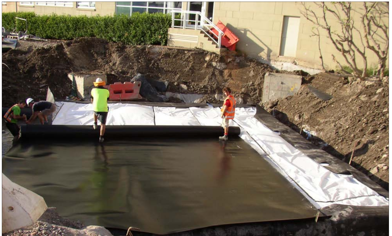
The tank wrapped in Geotextile and pulling the impermeable liner on top.
