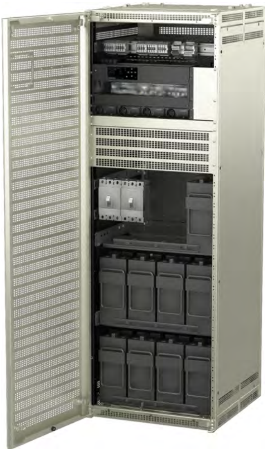
IBB SYSTEM IN FPC CABINET
