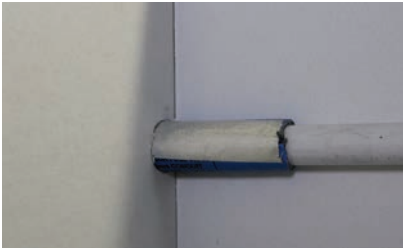
FIROBLOK CONDUIT SLEEVE FITTED INTO A 20MM COUPLING
