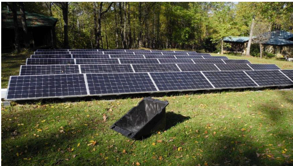
Figure 2. PowerField PV Solar Array
