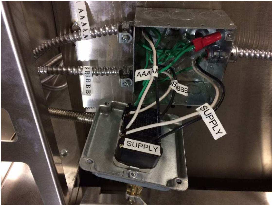
MAIN ELECTRICAL BOX SHOWING SUPPLY LINE ENTERING ON RIGHT SIDE OF BOX.
