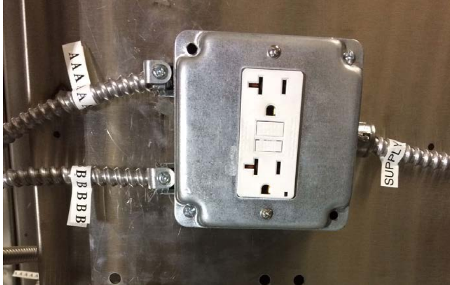
MAIN ELECTRICAL BOX COMPLETE
