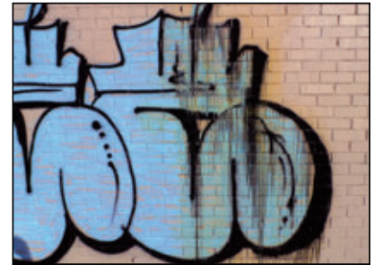
After applying BBSM, graffiti will start to run down the wall
