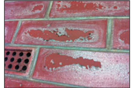
'Anti-graffiti' coating peeling/delaminating
