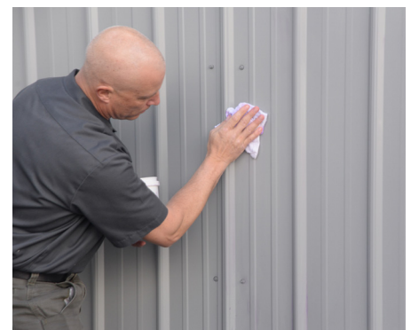
AFTER: This surface was cleaned with GRS non-toxic solution and in a few minutes, looked like new with no coating damage.
