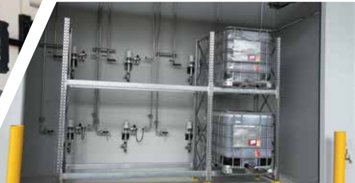
IBC Workshop Lubrication Distribution System
