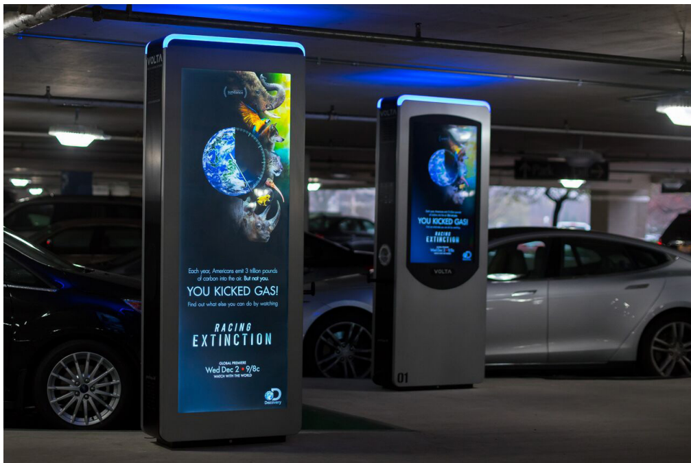
Volta Charging Stations installed in Oak Brook Center's Parking Garage in Oak Brook, IL
