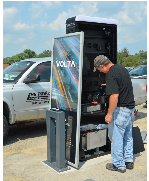
JNS Power & Control Solutions installing a Volta charging station in Oak Brook, IL
