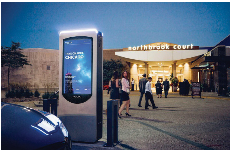
By fall 2015, 10 Volta charging stations had been set up across three locations in Illinois, including at the parking lot of Northbrook Court in Northbrook, IL.
