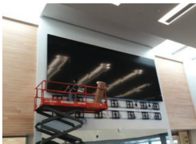
Integrator High-Tech Electric employed Peerless-AV's DS-VW755S Full Service Thin Video Wall Mount with Quick Release to create a 49-display Barco video wall high up in UC Riverside's new Student Recreation Center.
