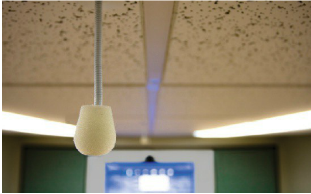
The Earthworks IM Installation Series gooseneck series were installed for enhanced intelligibility.
