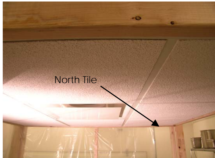
Figure 4: Air diffuser set-up: Centered air vent with eight surrounding 2' X 2' ceiling tiles
