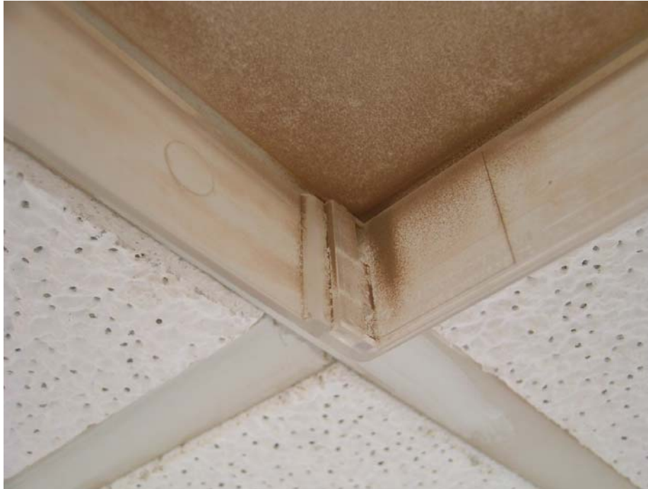
Figure 18: Dust accumulation in North East Corner of deflector
