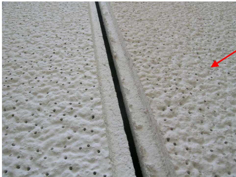
Figure 19: South edge of the north tile (location of deflector) after exposure (right)
