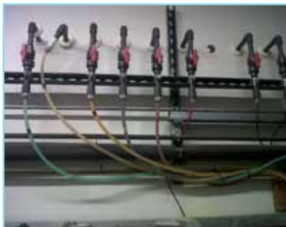
CUSTOM-CONFIGURED WATER MANAGEMENT/DISTRIBUTION SYSTEM
