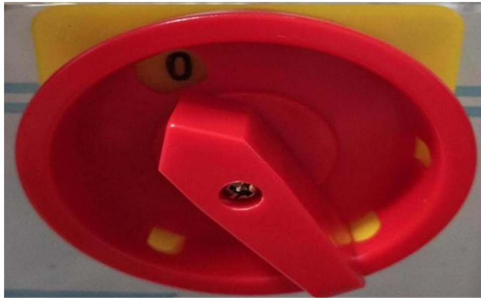
Picture 4: Power switch
