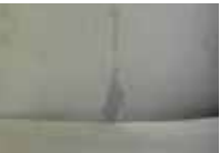
Indoor water damages
