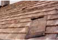
Building structure degradation: mould and mildew
